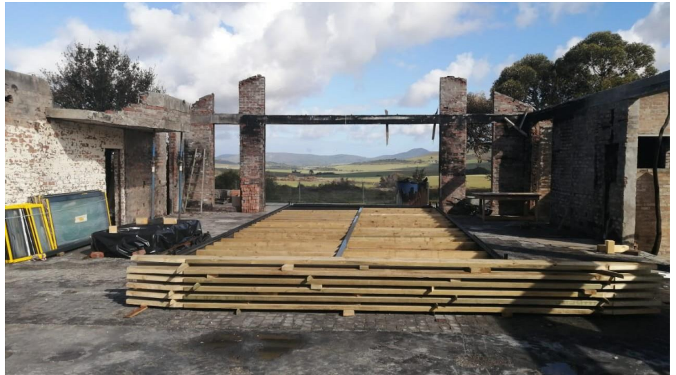
Our first project after the fire is the rebuilding of the "iMed clinic", here in the beginning stages. This is an open-air production and thereafter the workshop roof will go up.
